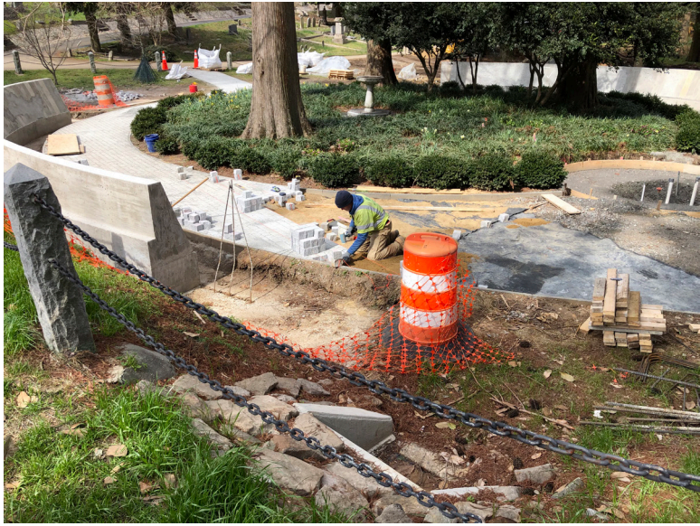
As fund raising continues, construction is underway on the Glade scattering garden at the entrance of Hollywood
