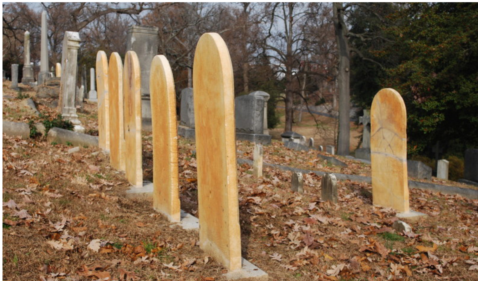
The back sides of the Norton family plot tablets as they appear today. There is clear evidence of orange staining brought about from years of direct exposure to the ground. Section D, Plot 204. See page 1.
